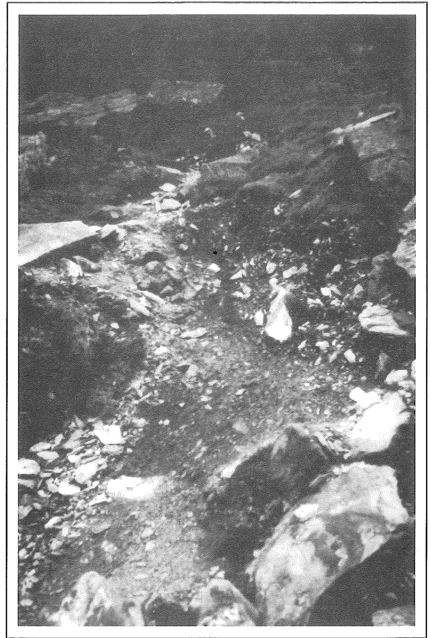
A badly-eroded surface susceptible to severe storm damage
